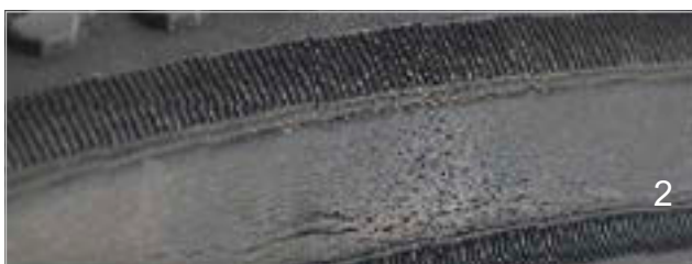
Figure 50: Examples of fatigue cracks (1) and ageing cracks (2)
